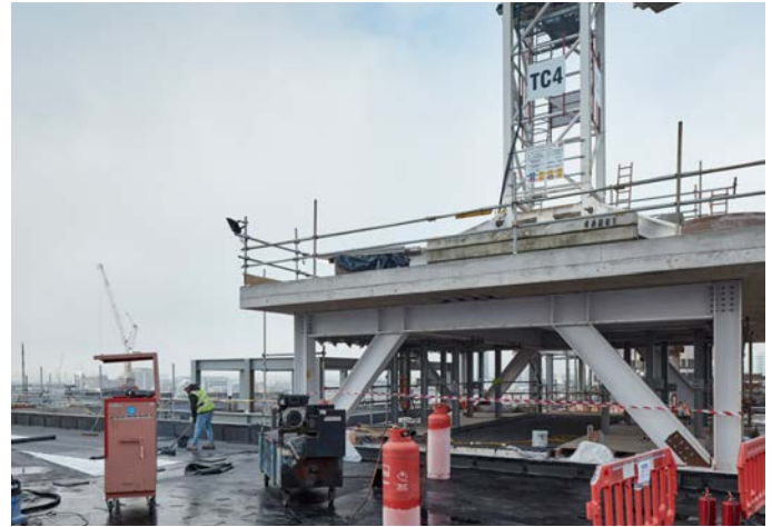
opposite: Level 06 terrace and 'martini' transfer column above: L10 communal terrace bottom: L10 communal terrace
